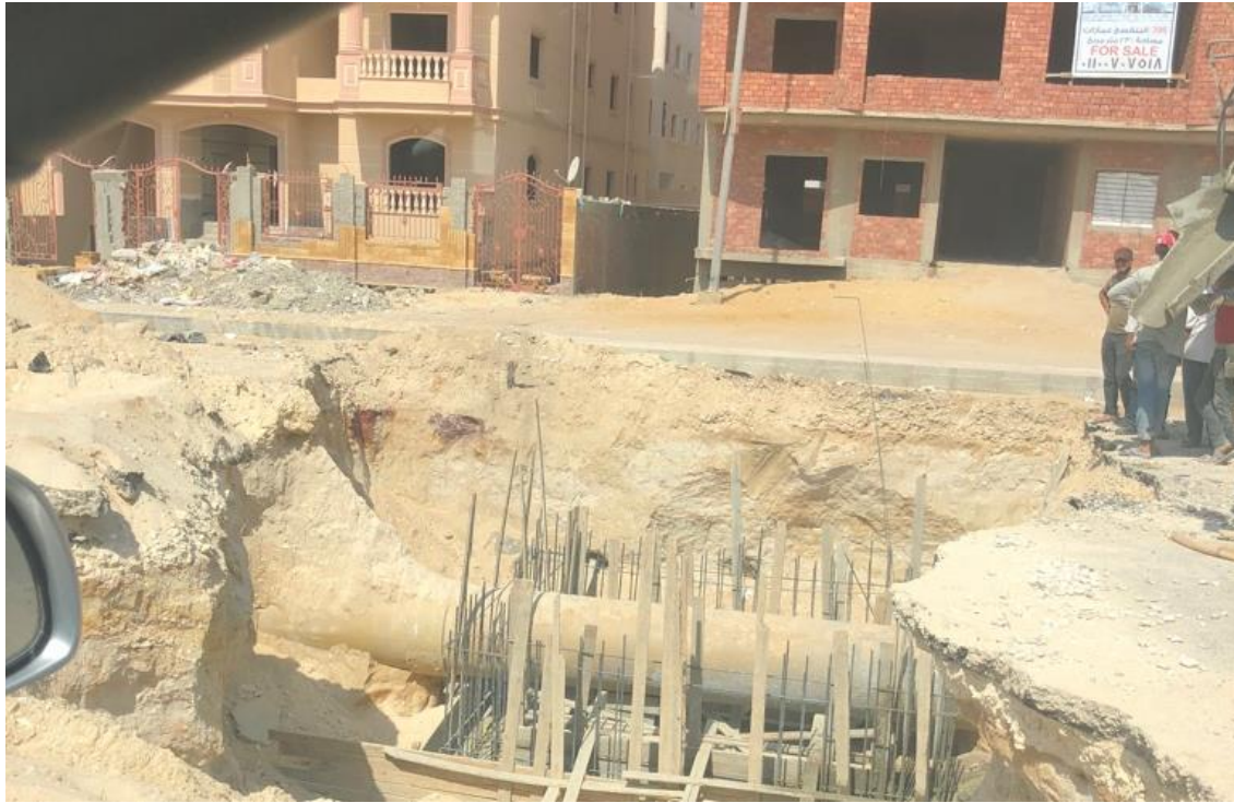
Figure 46: An underground pipe with construction supports. October 2018
