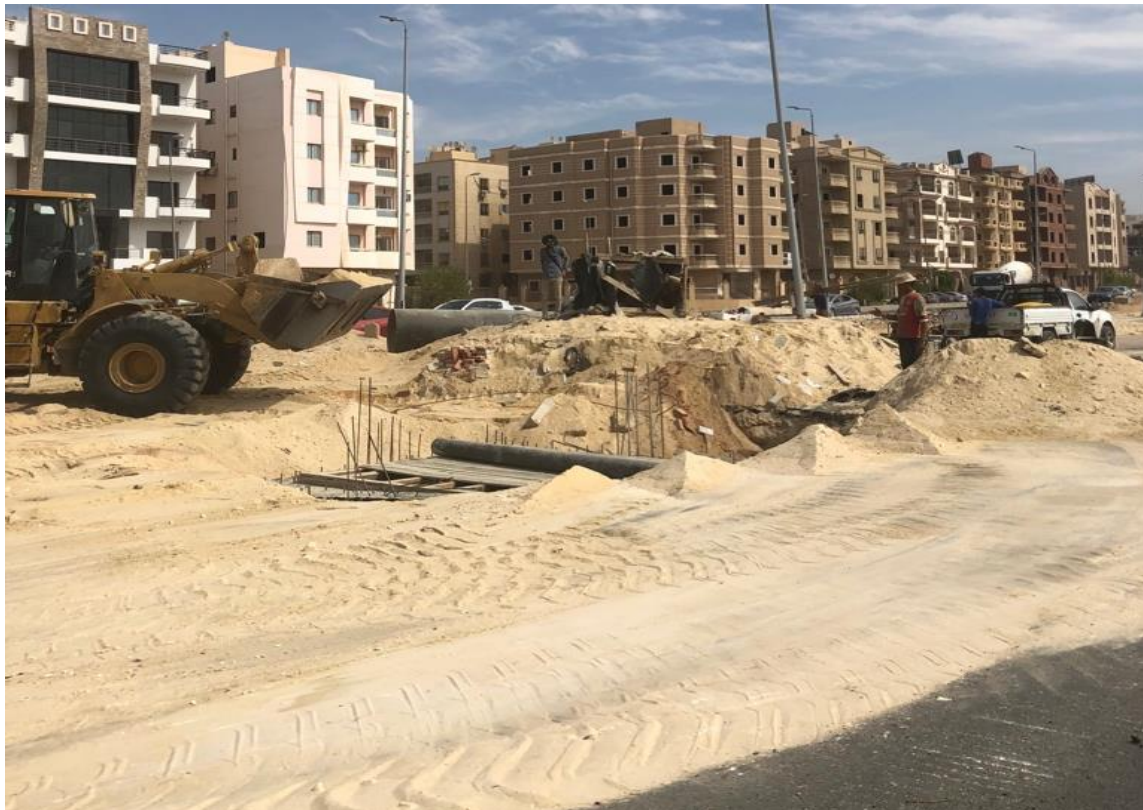
Figure 47: More pipes were installed in October 2018 after North 90 Street in was paved. Notice the new destroyed asphalt
