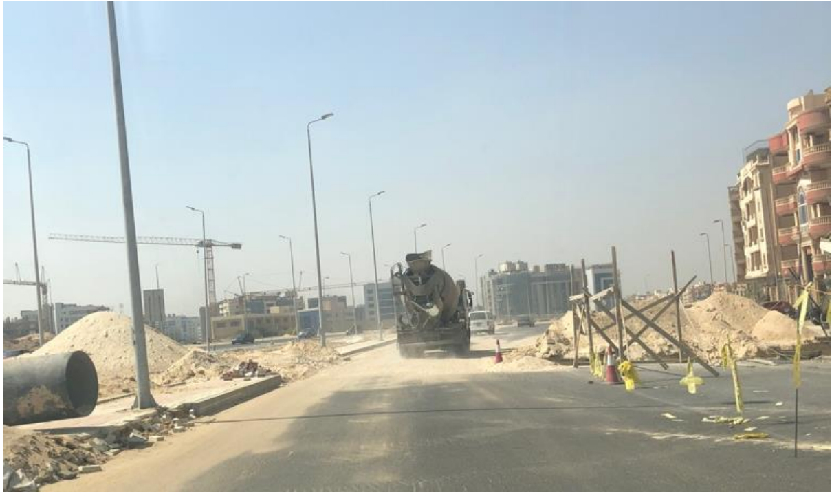
Figure 44: Underground Pipes are being installed and the new asphalt is destroyed in October 2018
