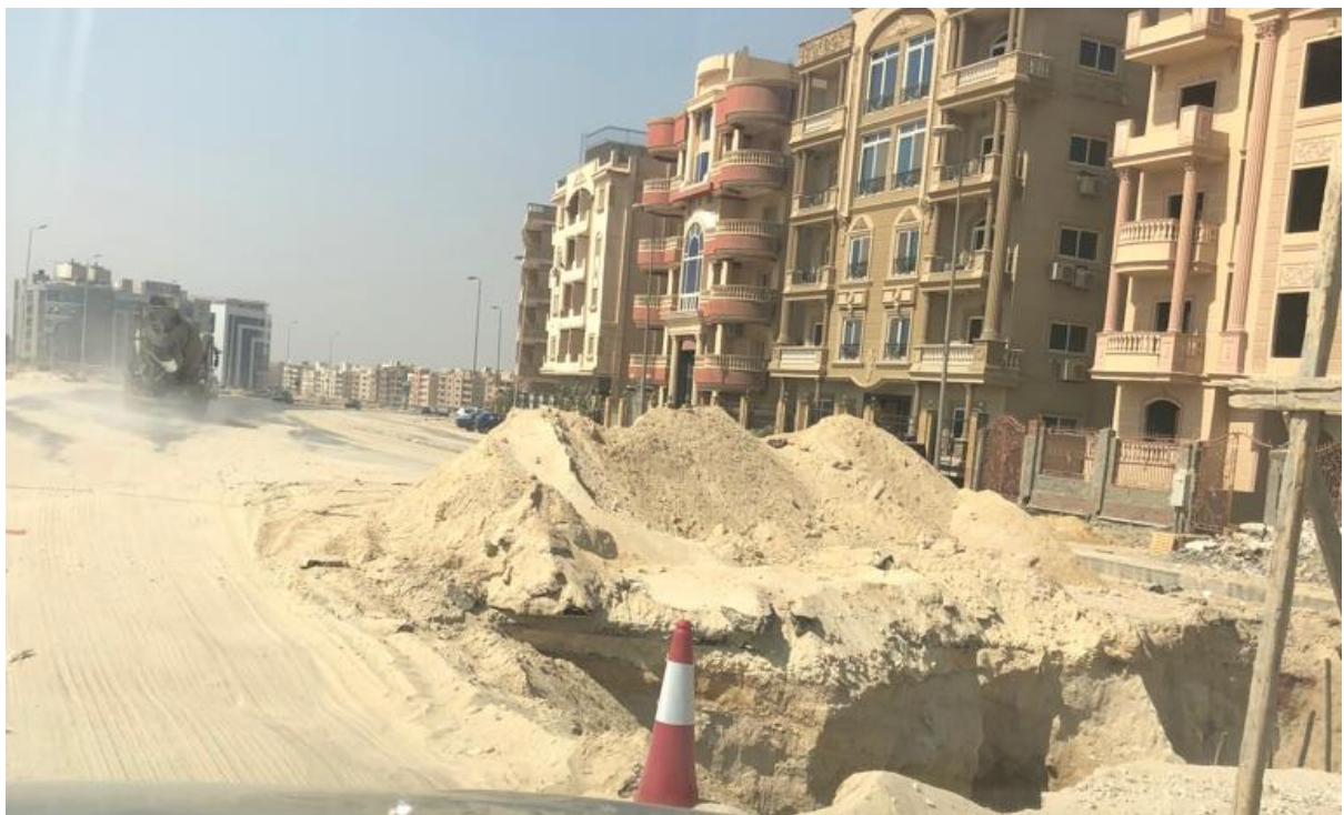
Figure 45: A closer look at the destruction of the newly paved North 90 road in October 2018
