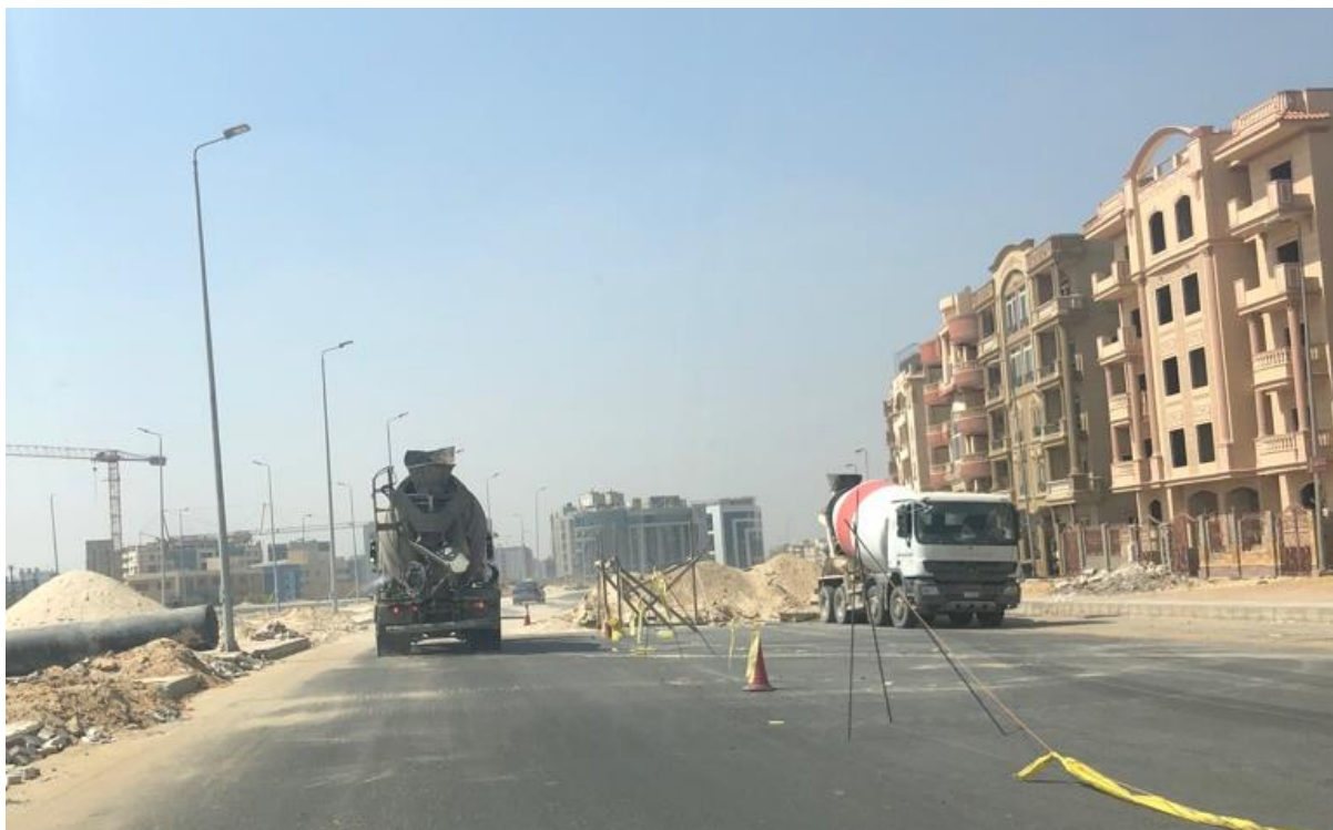
Figure 43: The Newly paved North 90 Street is being destroyed in October 2018
